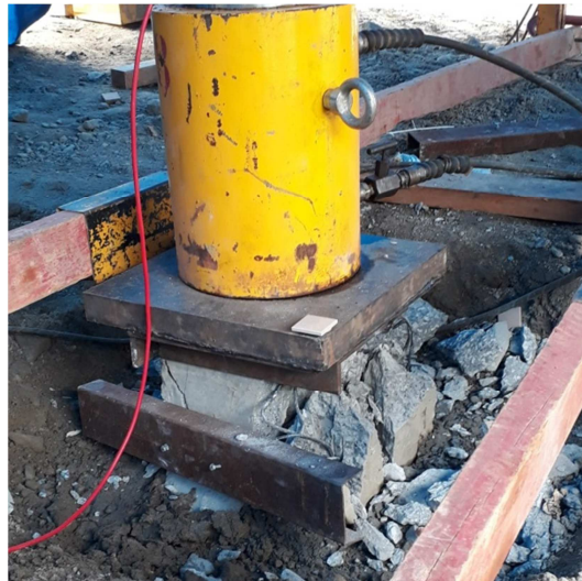
Figure 1. The pile ET01 broke when it reached a load of 242 tons.
