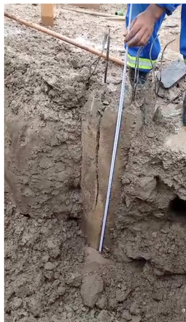
Figure 2. The extension of the damage on pile ET01.
